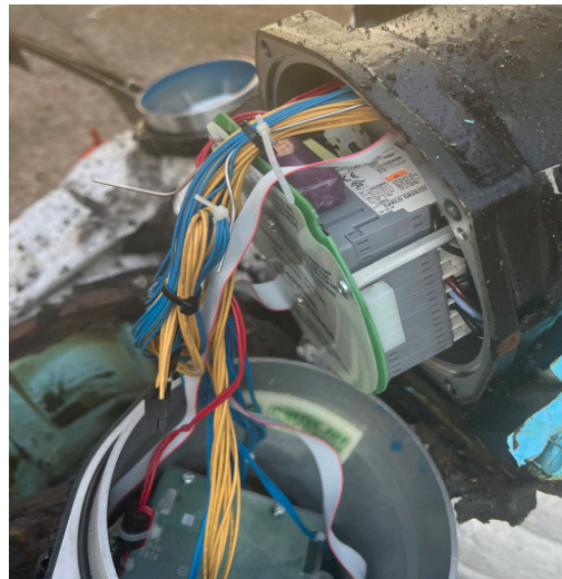
Electronics cover removed showing undamaged wiring, solder and printed circuit boards
